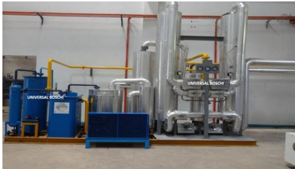
Process Skid (With Pre Cooling & Purification Unit)
