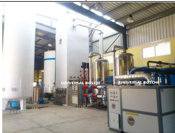
UBTL 200 Nm3/Hr (LIQUID OXYGEN TANK FILLING PLANT)
